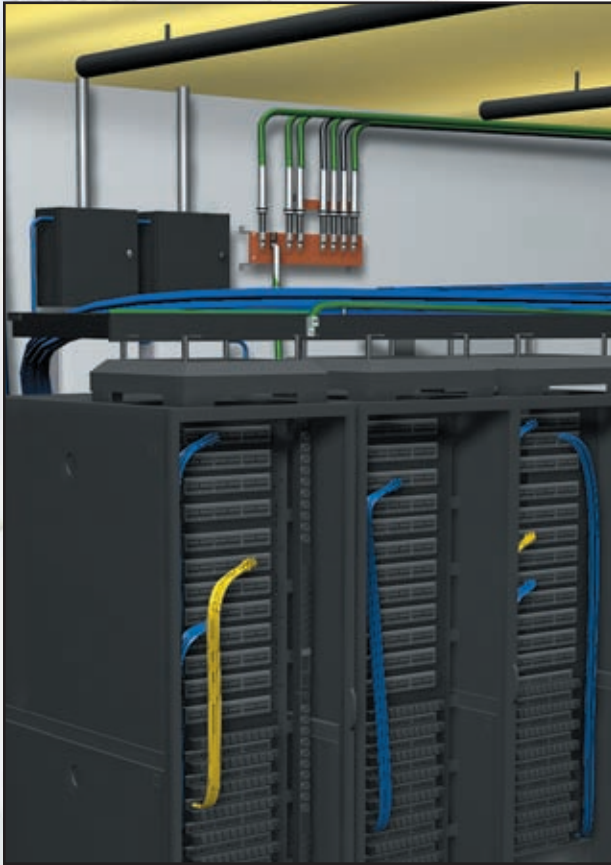
Grounding the ladder rack will help eliminate electrical signals that travel with cables.
