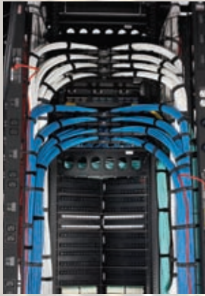
Separates horizontal cable from one rack bay to the next.
